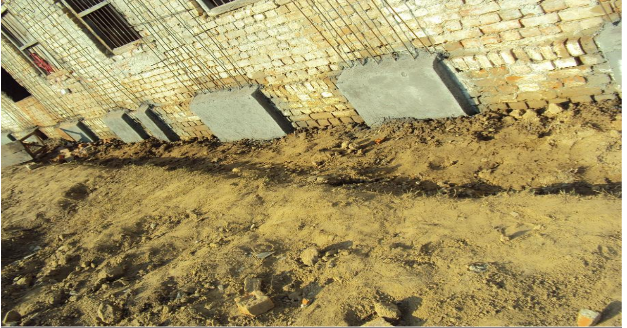
Splints upto Ground Level
