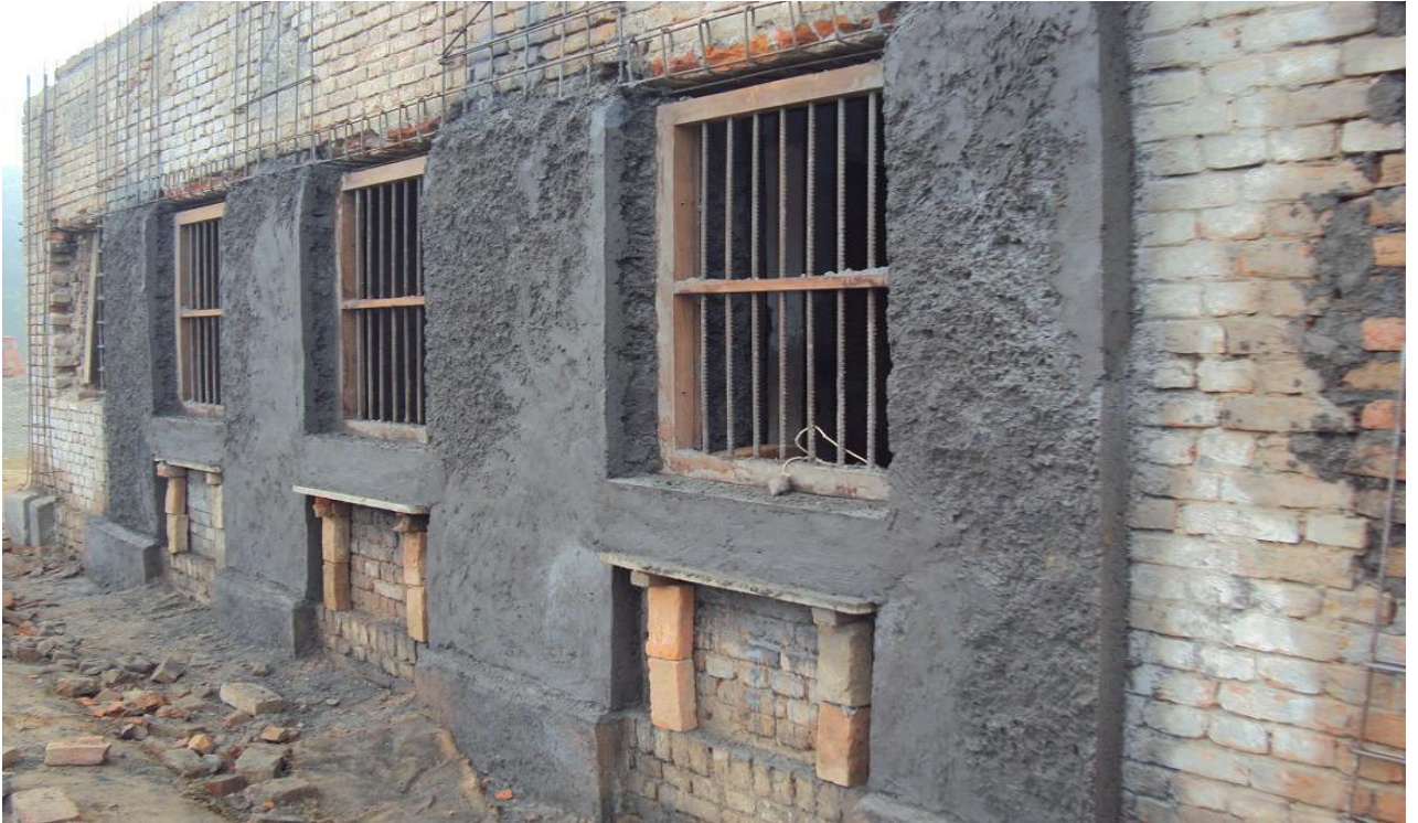
Micro Concrete Work of Splints and Bandage at Sill Level and Placement of New Windows
